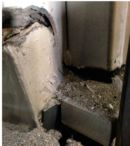
Figure 15 - Torn steel shell caused by the expansive reactions between backup materials and penetrated aluminum metal. The force exerted by crystal growth/expansion is very significant.
