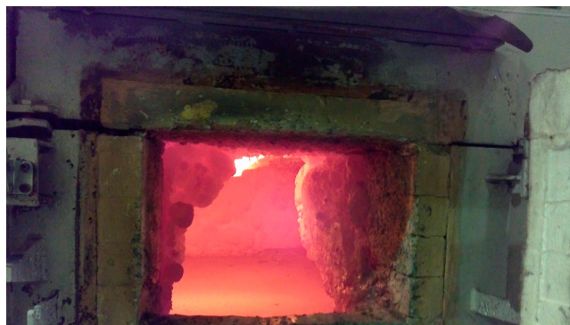
Figure 2 - Massive corundum formation near door area of melter. This cannot be removed at this point without significantly damaging the remaining lining.
