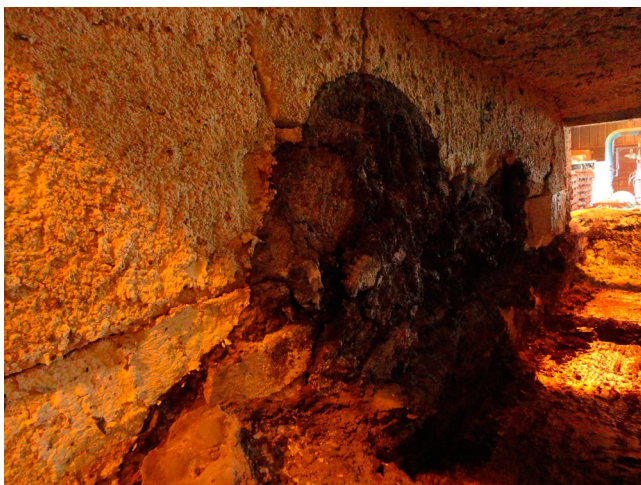
Figure 7 - Penetration and Conversion of a large portion of the upper and lower sidewalls of a melting furnace. The lower sidewall is heaved out significantly.
