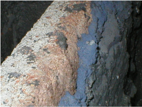
Figure 1. Corundum build up on refractory sidewall.
